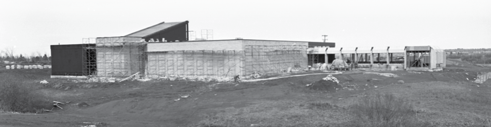
Construction of Rt. Hon. J.G. Diefenbaker Centre underway, 1979. Courtesy University of Saskatchewan Archives & Special Collections, A-8923.
